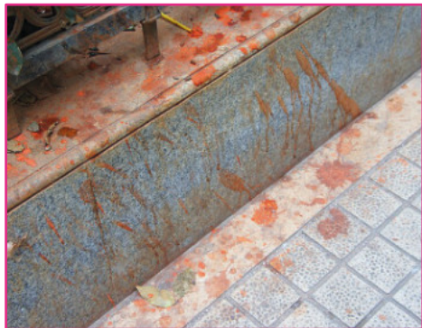
Staining caused by spitting Paan
